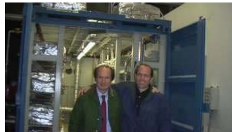
Here I am with Andrea Ross after the test of the 1 MW E-Cat plant in the background.
