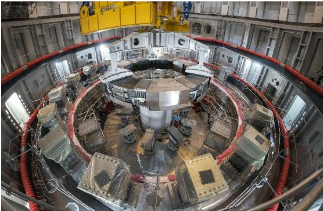
PHOTO CAPTION: This photo shows the installation of the first superconducting magnet, Poloidal Field Coil #6, in the tokamak pit at the ITER construction site. The Central Solenoid will be mounted in the center after the vacuum vessel has been assembled. Courtesy ITER Organization.
