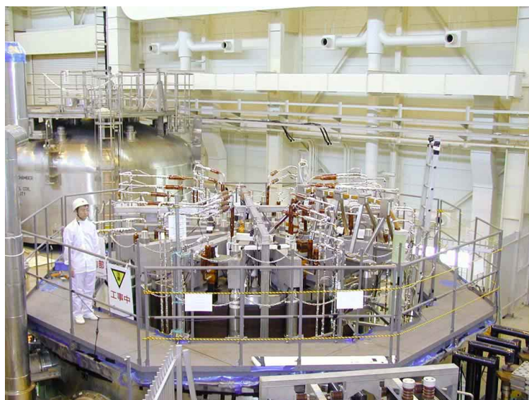
Figure 2.1.10-1 CS Model Coil and CS Insert Installed in the Vacuum Chamber at the Test Facility in JAERI Naka
